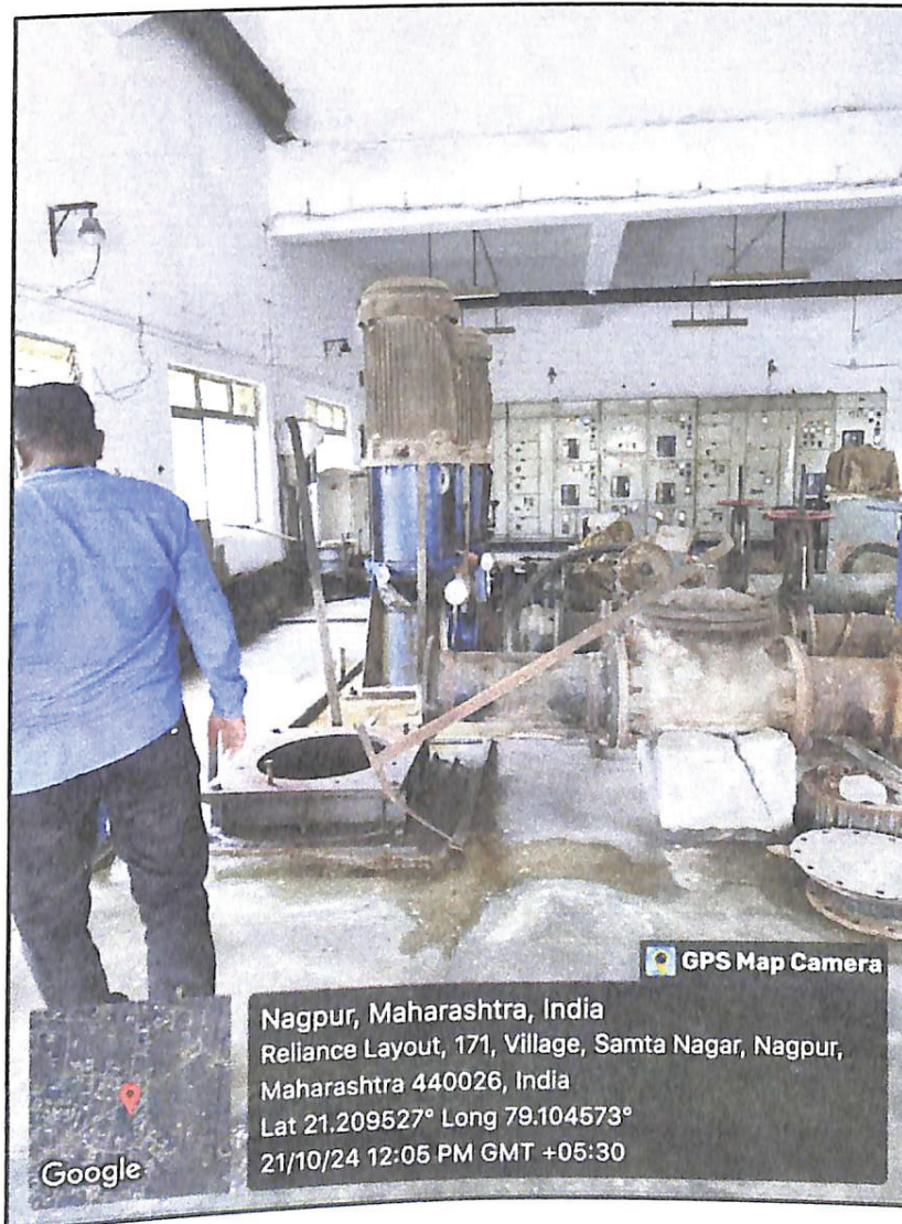
Figure 6: Ash water recovery pump house
