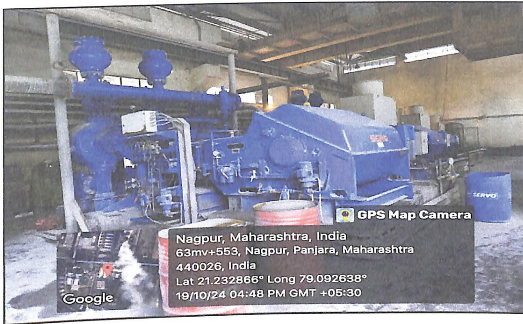
Figure 3: Dry fly ash slurry discharge pumps
